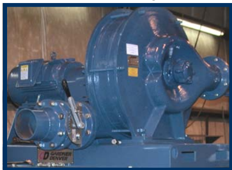
Exaustor Gardner Denver 4203A e motor de 20 HP no filtro Vac-1000
